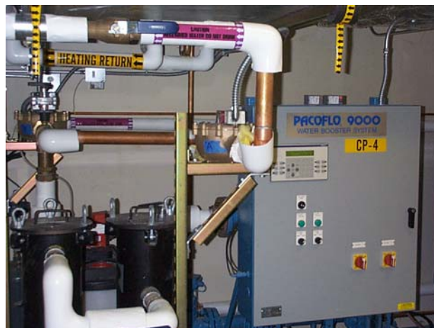
Rainwater Harvesting System
